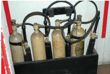
One of several sets of original fire extinguishers
